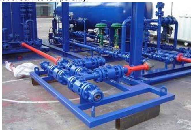
Figure 172 Oil and Gas Manifold
